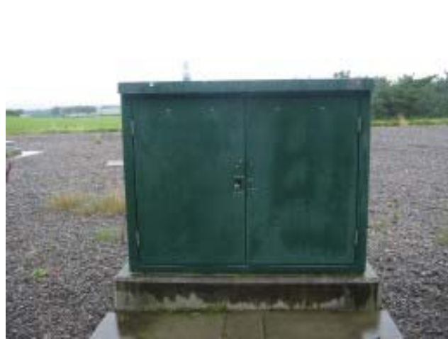
Equipment Cabinet Mounting #2.
