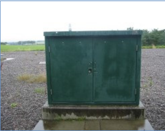
Equipment Cabinet Mounting #2
